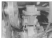
18.1 View of vacuum pump with oil cleaner removed showing fillerhead plug (arrowed)
